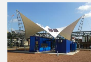
PemGen commissioning Support
